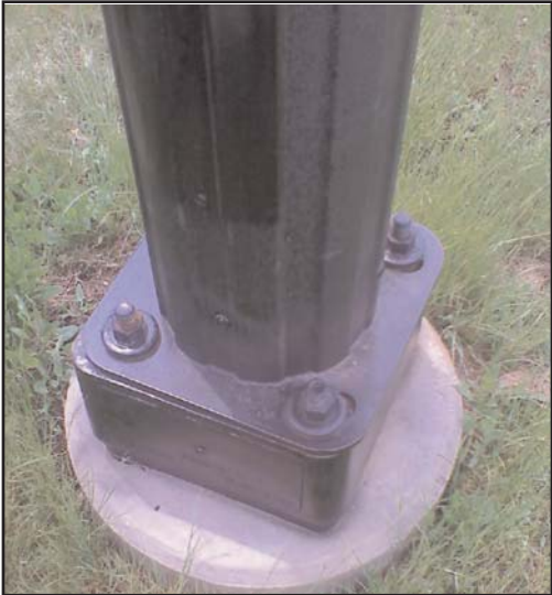
Duratel light pole installed on legacy base
